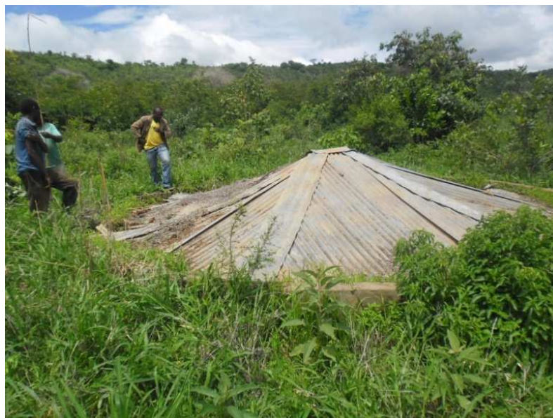
Figure 4: A neglected underground tank (Source: Author, January 2015)
