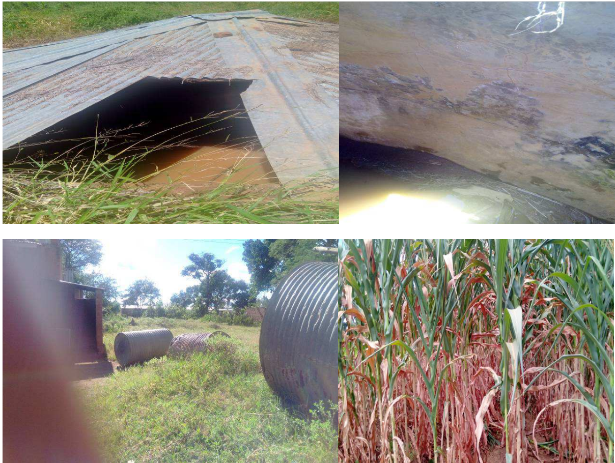
FIG 2: Photos of water harvesting tanks in Bolero, EPA Top right: A dilapidated roof top of an IRLAD supported water tank in Bata Section, Top left: Inside the cracked leaking water tank, Bottom right: Abandoned water harvesting tanks at Bolero EPA and Bottom left: A scorched maize crop in a farmers fields 100 meters away.
