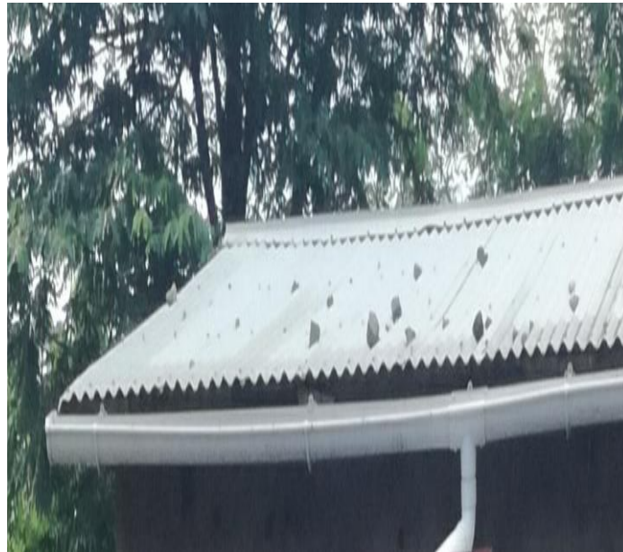
Roof catchment and supporting collecting
